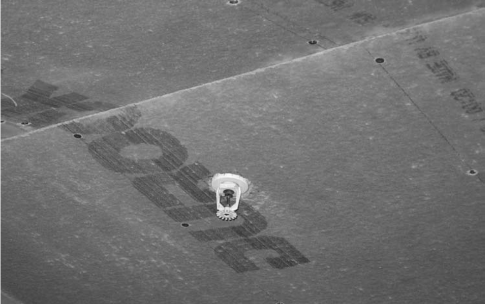
Ceiling (with sprinkler head) showing Tile Council of North America (TCNA) recommended pitch of 2" per foot (50 mm per 300 mm).
