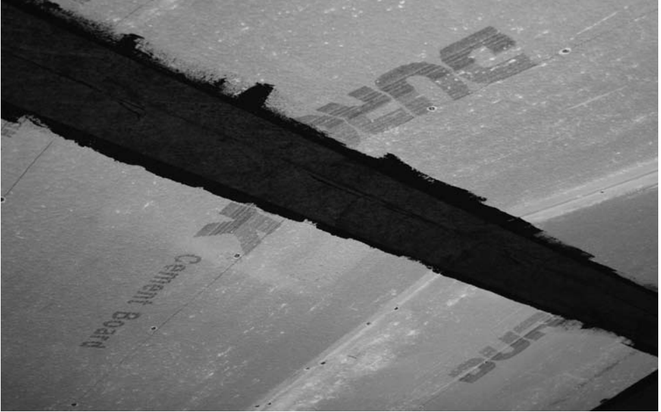
Pre-treatment of ceiling joint with 6" (150 mm) wide, treatment of LATICRETE 9235 Waterproofing Membrane.
