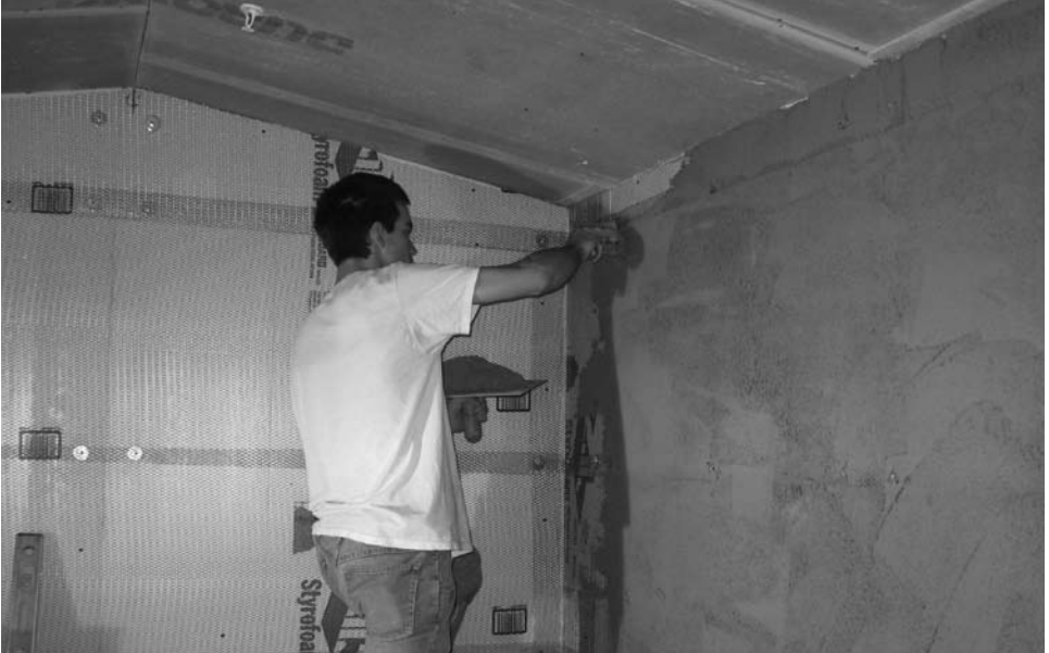
Finishing the application of the LATICRETE 226 Thick Bed Mortar and LATICRETE 3701 Mortar Admix scratch coat.
