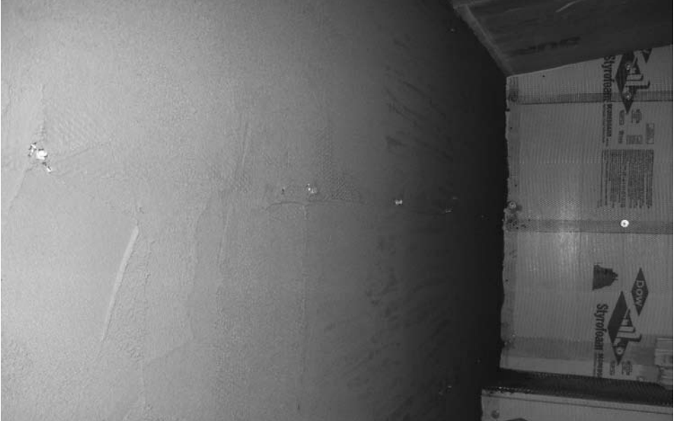
A finished, scratch coat wall which is now ready for “the float coat.”
